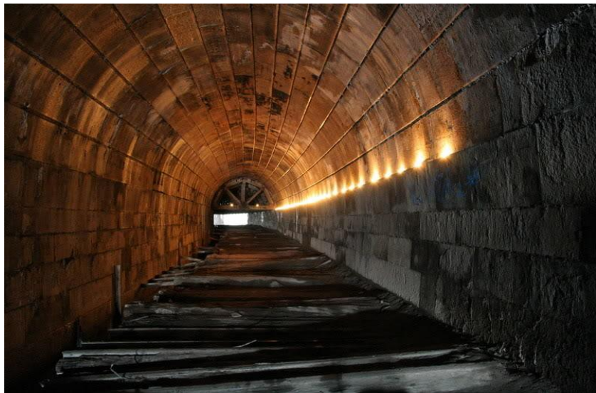
Figure 18. Old Merritton Tunnel built in 1800s and is no longer in use.
